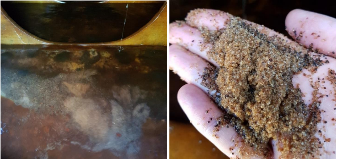
Figure 3-7: Filter sand and coal found in filter underdrain
