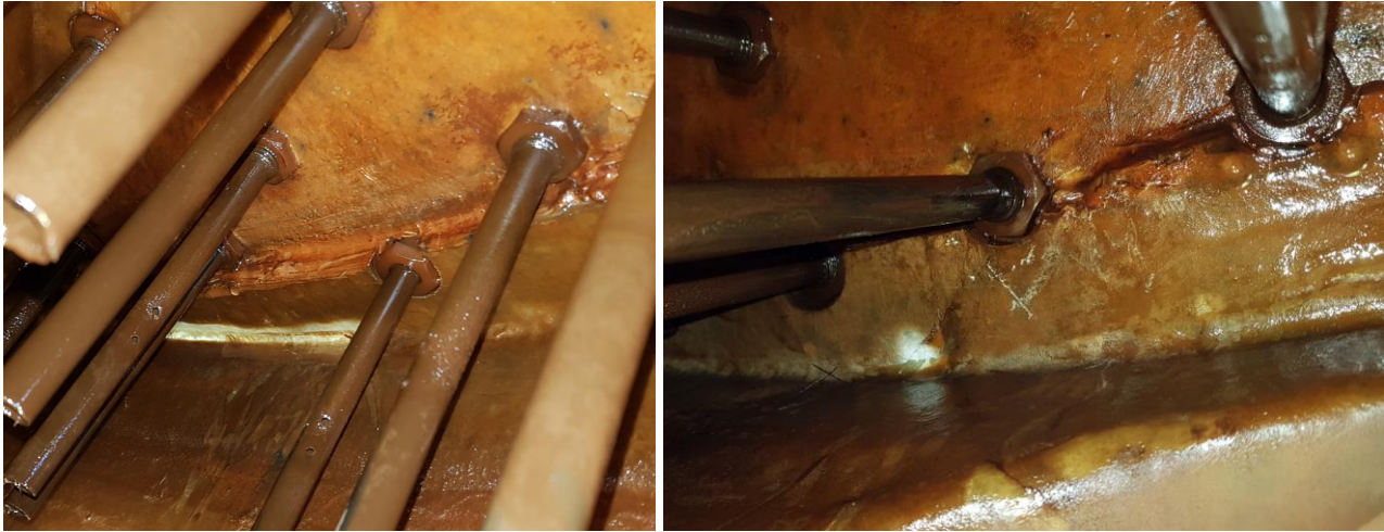
Figure 3-9: Underdrain floor joint failure and cracking
